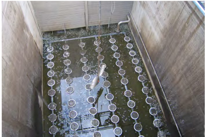
Denitrification can be an intermittent aeration process with anoxic and aerobic phases created alternately.
